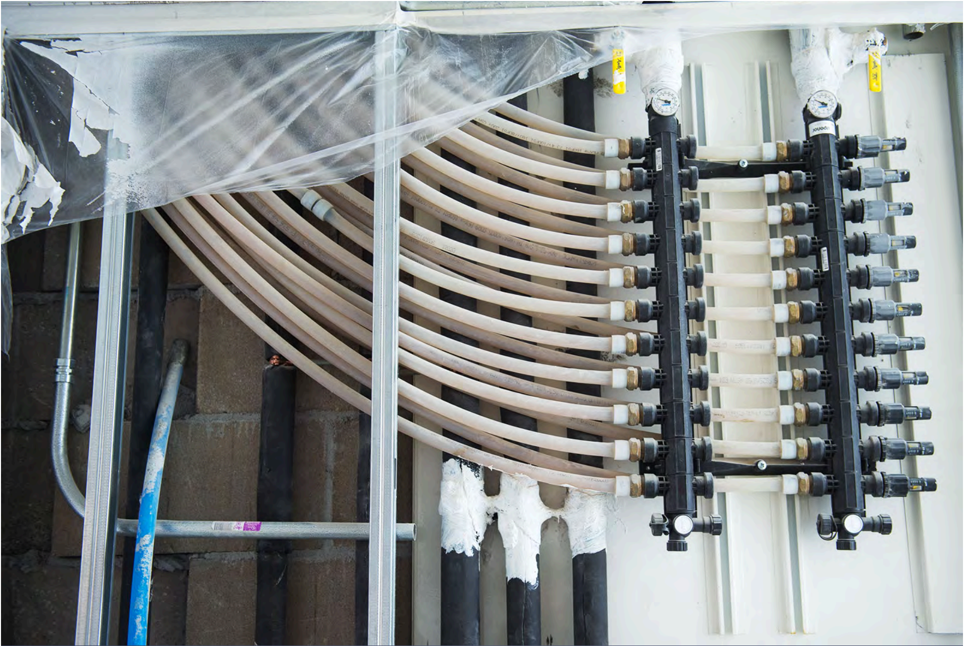
Cast in tubing for radiant heating and cooling
